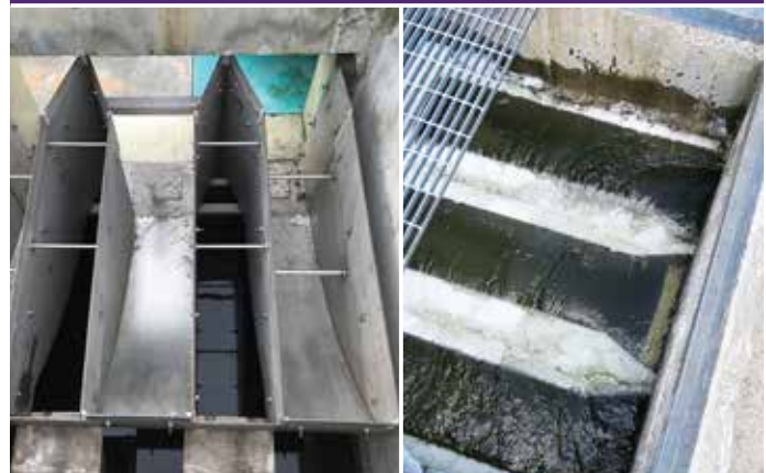
SERPENTINE WEIR CONTROLS
