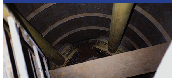
View into central valve access and waste drain column, showing individual cell waste valves and actuators.
