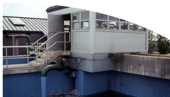
QuadraKleen™ unit, showing optional control room.
