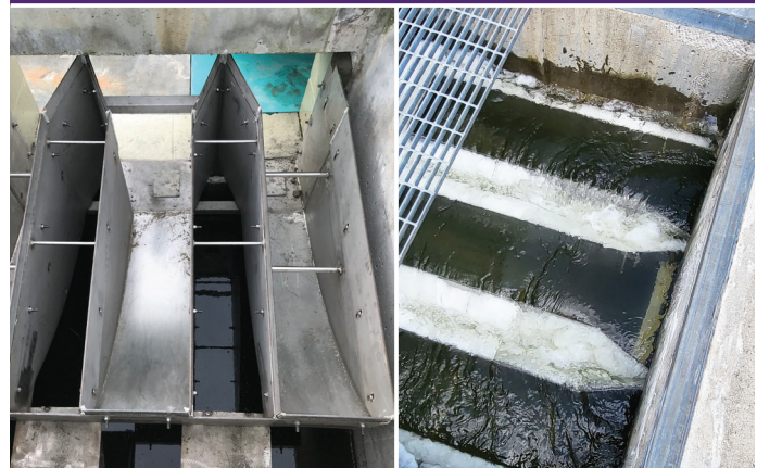
SERPENTINE WEIR CONTROLS
