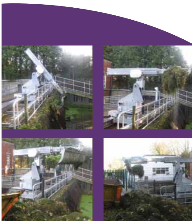
Brackett Bosker® Bandit automatic trashrake debris being dumped directly into containers for waste treatment or recycling.
